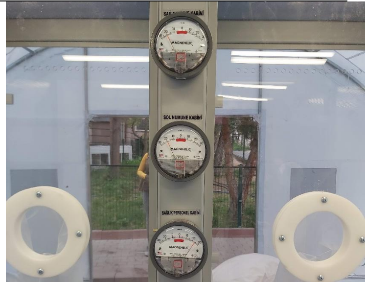
Figure 5 Pressure Manometer in The Cabinet Rooms
